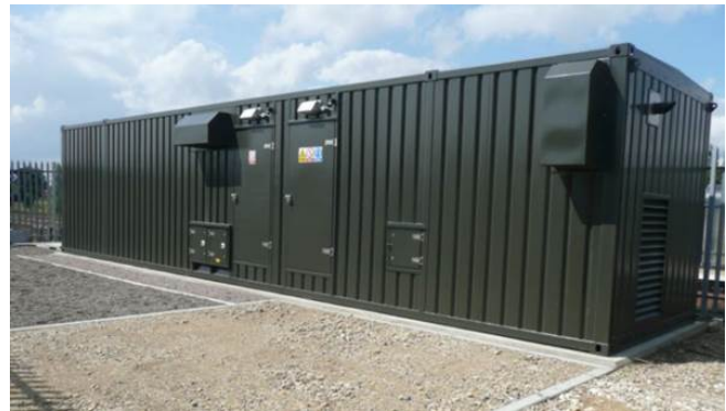
Plate 4.3: Example of a principal supply point
