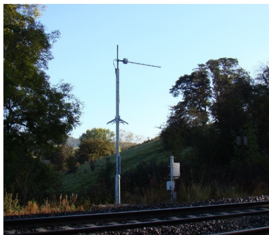
Plate 4.7: A typical pole mounted GSM-R repeater
