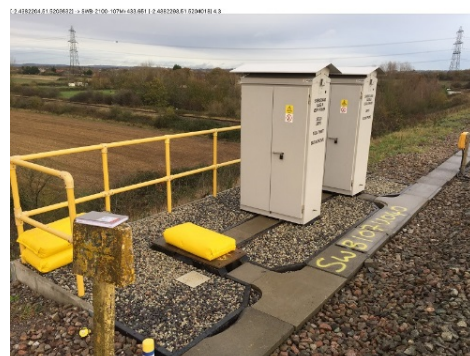
Plate 4.6: An example of LOC Cabinets
